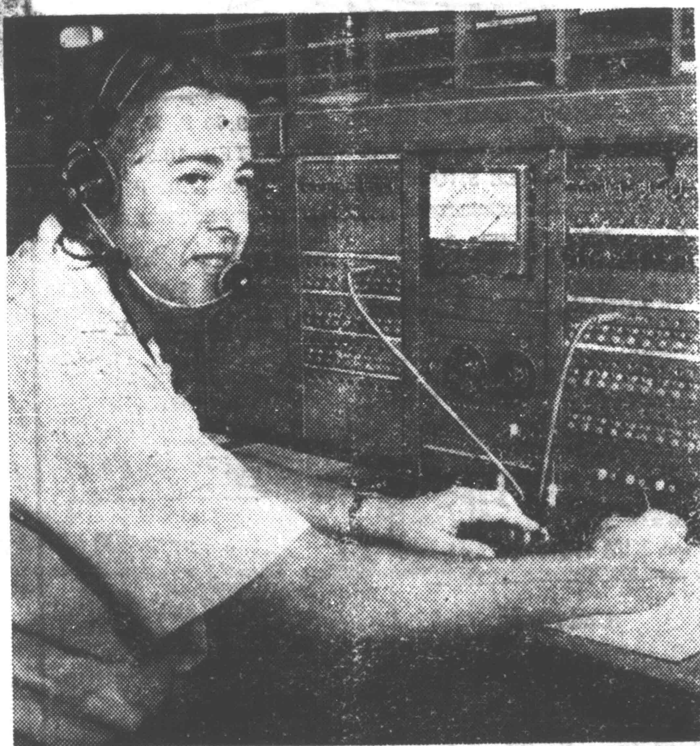
Guided by electronic "eyes and ears," the test deskman spots line troubles at once and gets repairs there quickly, often before service is actually interrupted.
